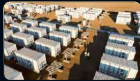
400MW + 1.3GWh Saudi Arabia, 2023
