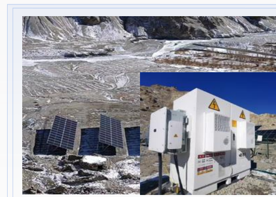
Off-grid power supply @ china High altitude
