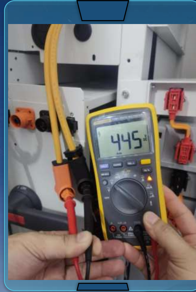
Measurement of tower voltage
