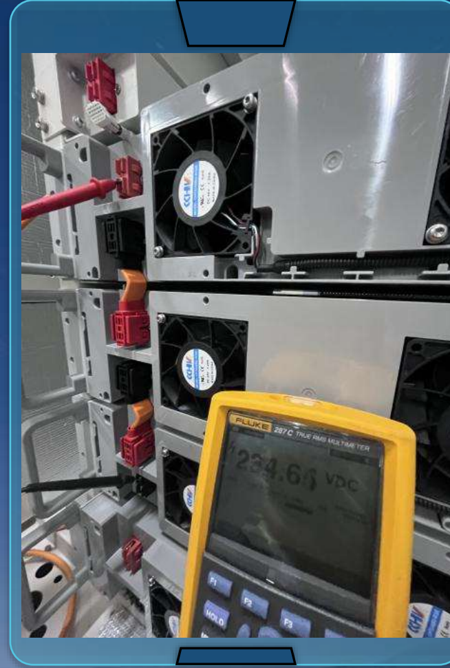
Multiple Module Measurement
